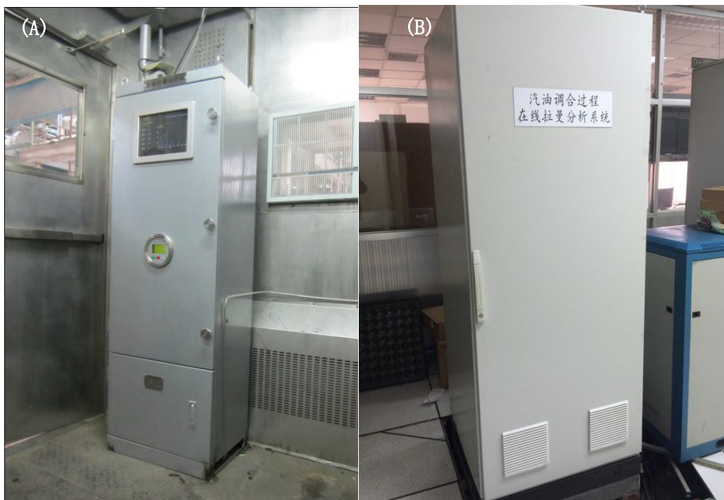
Figure 5. Main cabinet of analysis system:
