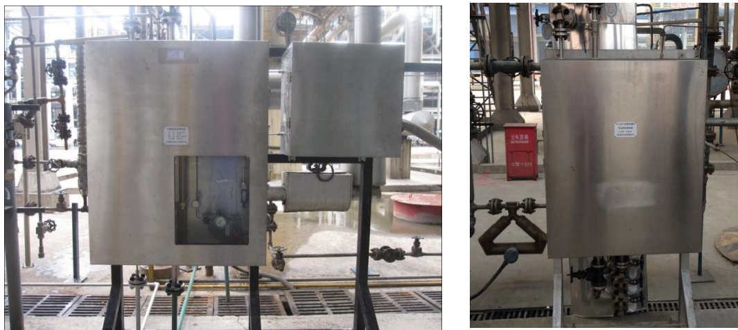
Figure 4. On-site sampling cabinet of Analysis system
